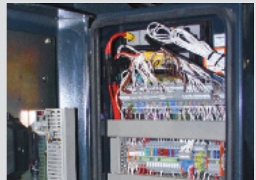
Centralized electrical panel allows systematic and efficient trouble shooting.
