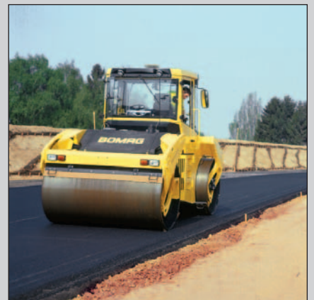
Large-scale asphalt work requires highly efficient rollers: BW 203 AD with ASPHALT MANAGER.
