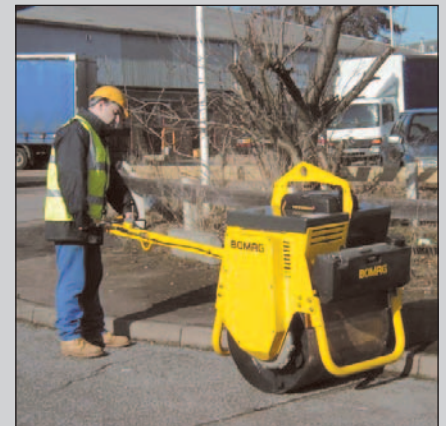
Standard with water sprinkler system.
