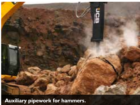
Auxiliary pipework for hammers.
