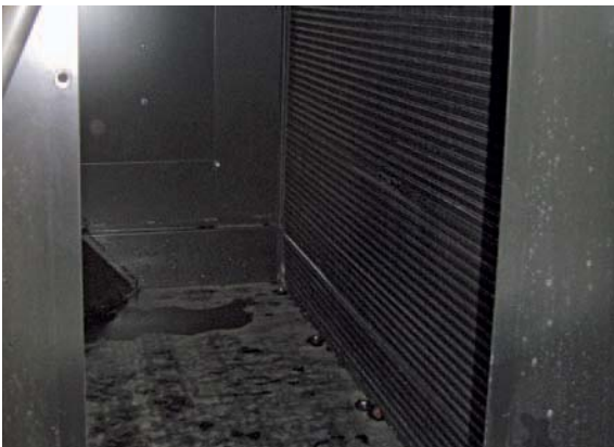
Excellent access for cooler cleaning.
